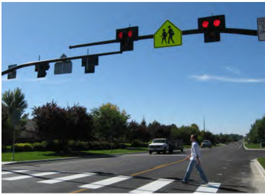
PEDESTRIAN HYBRID BEACON AT CROSSWALK
